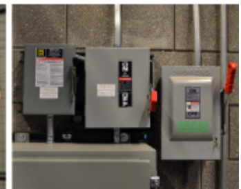
HIGH VOLTAGE RISK
